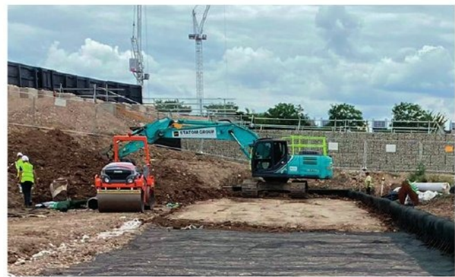
Top: The site was previously occupied by Barking Power Station which was decommissioned in 1981 Bottom: The site was underlain by a layer of peat that had to be removed before work on the wall foundation could begin
