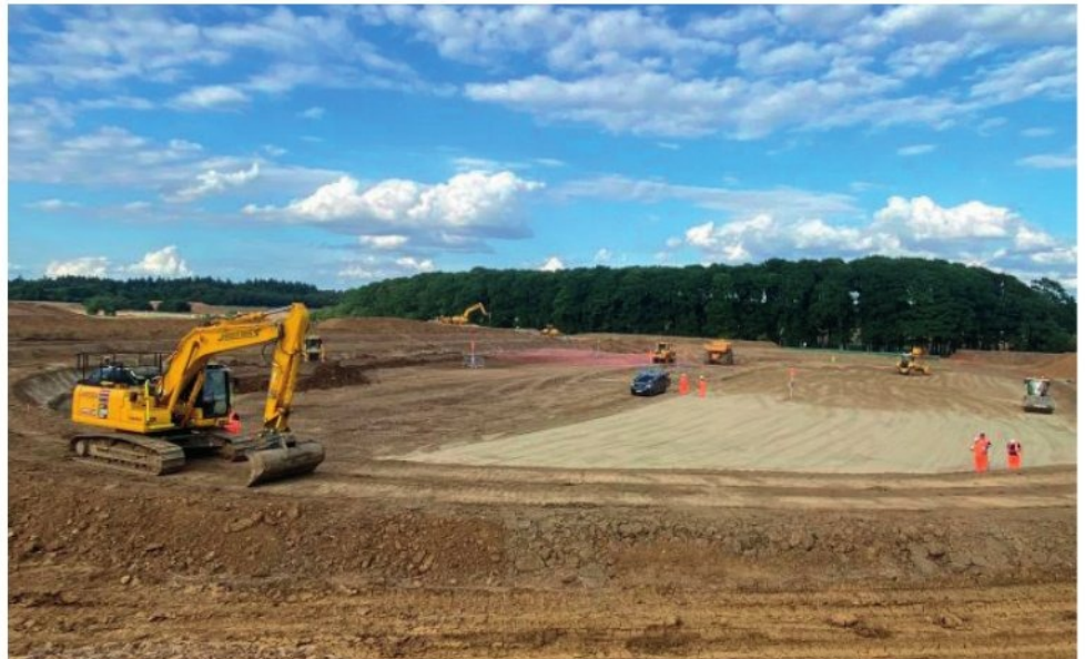
Main construction work for the Havant Thicket Reservoir in Hampshire is expected to start next year
